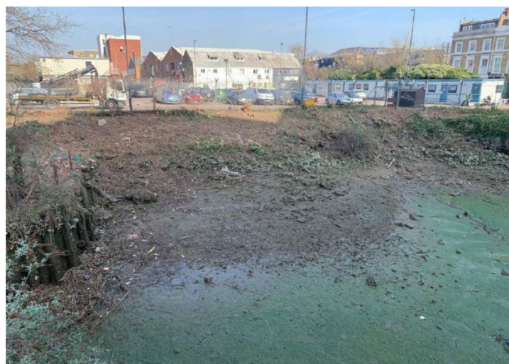
Current condition of the creek wall, with back-filled section between the walled sections clearly visible.
