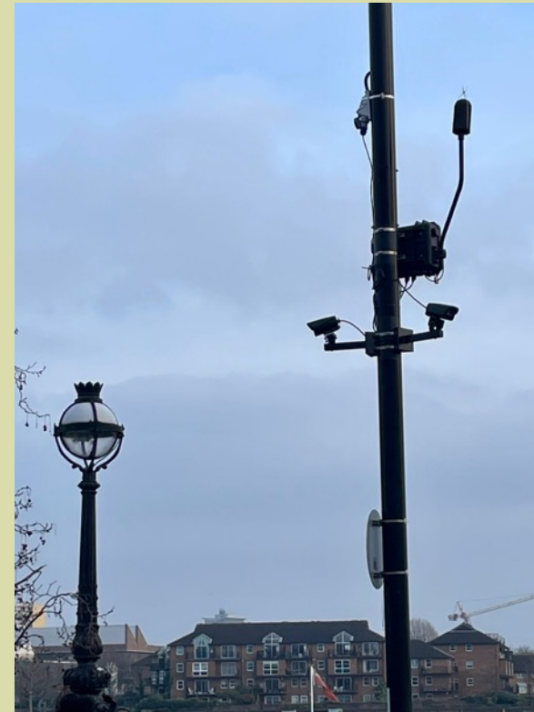
Acoustic Camera installed on Cheyne Walk
